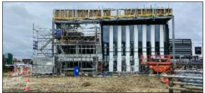
WORK IN PROGRESS: The new dining hall still has a way to go for completion.
