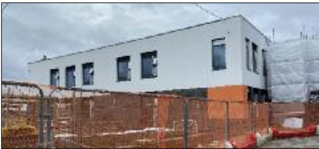
TAKING SHAPE: The new Science and Food Technology block is well under way.
