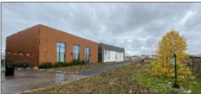
ON TRACK: The new performing arts centre next to the existing music block.
