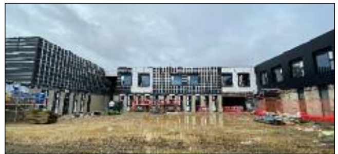
SIXTH FORM BUILD: The new facilities for post-16 study will be ready for September 2024 when the sixth form opens.
